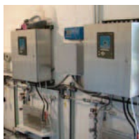
Field remote terminal.
