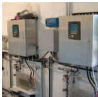
Field remote terminal.
