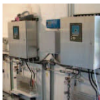
Field remote terminal.
